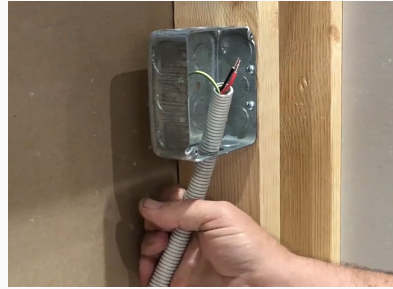
2. Pull 90C wire (Hot, Neutral, Ground) to the Junction Box with a 6" loop
